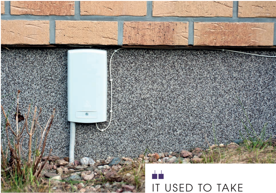
Computer vision AI can be leveraged to check the quality of the splicing in the wall box outside the customer's premises
